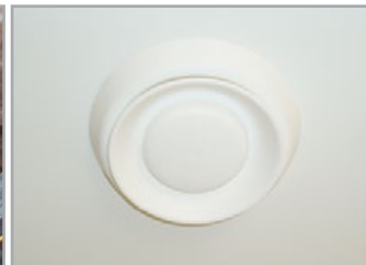
Finished installation with Primex WG Series Diffuser
